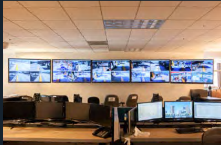
CCTV monitoring at the BOC
