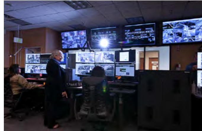
CCTV monitoring at the ROC
