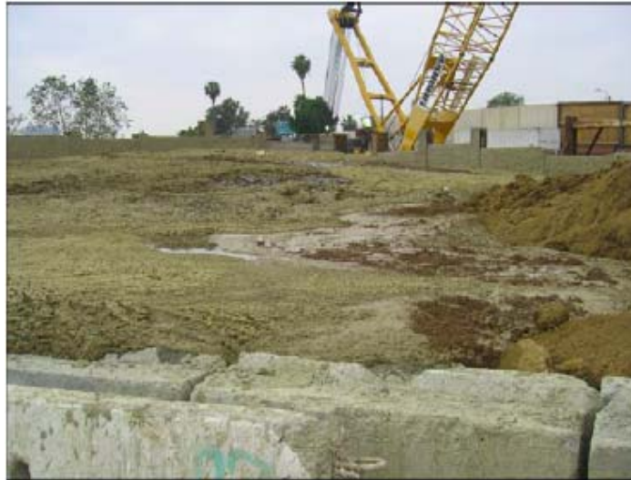
Figure 4-1: Wet Soil at Surface EPB TBM
