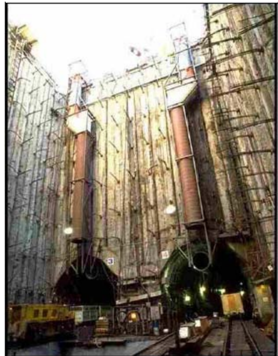
Draft Environmental Impact Statement/Environmental Impact Report Figure 2-4. Secant Pile Wall for the Barnsdall Shaft in Hollywood
